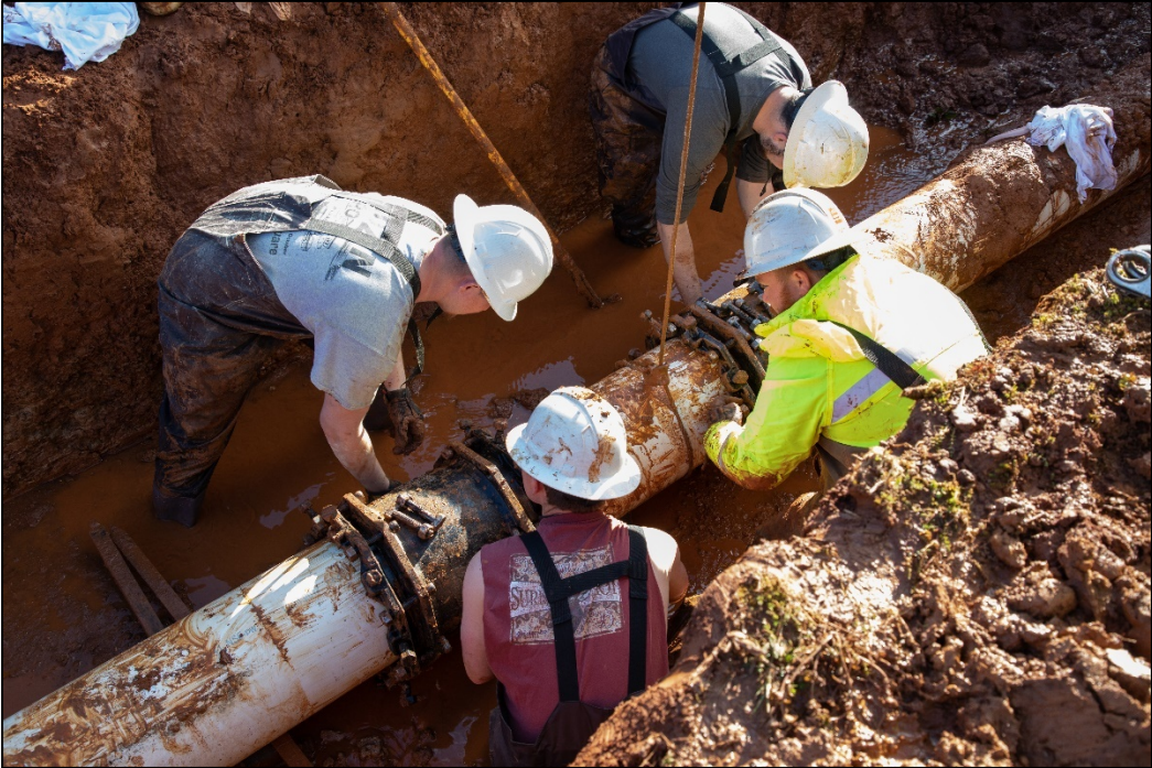
Huntsville Utilities Water crews working as a team on a service main break.
